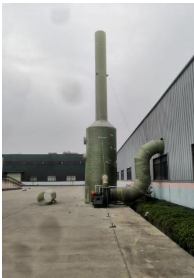
喷淋塔+15m 排气筒
